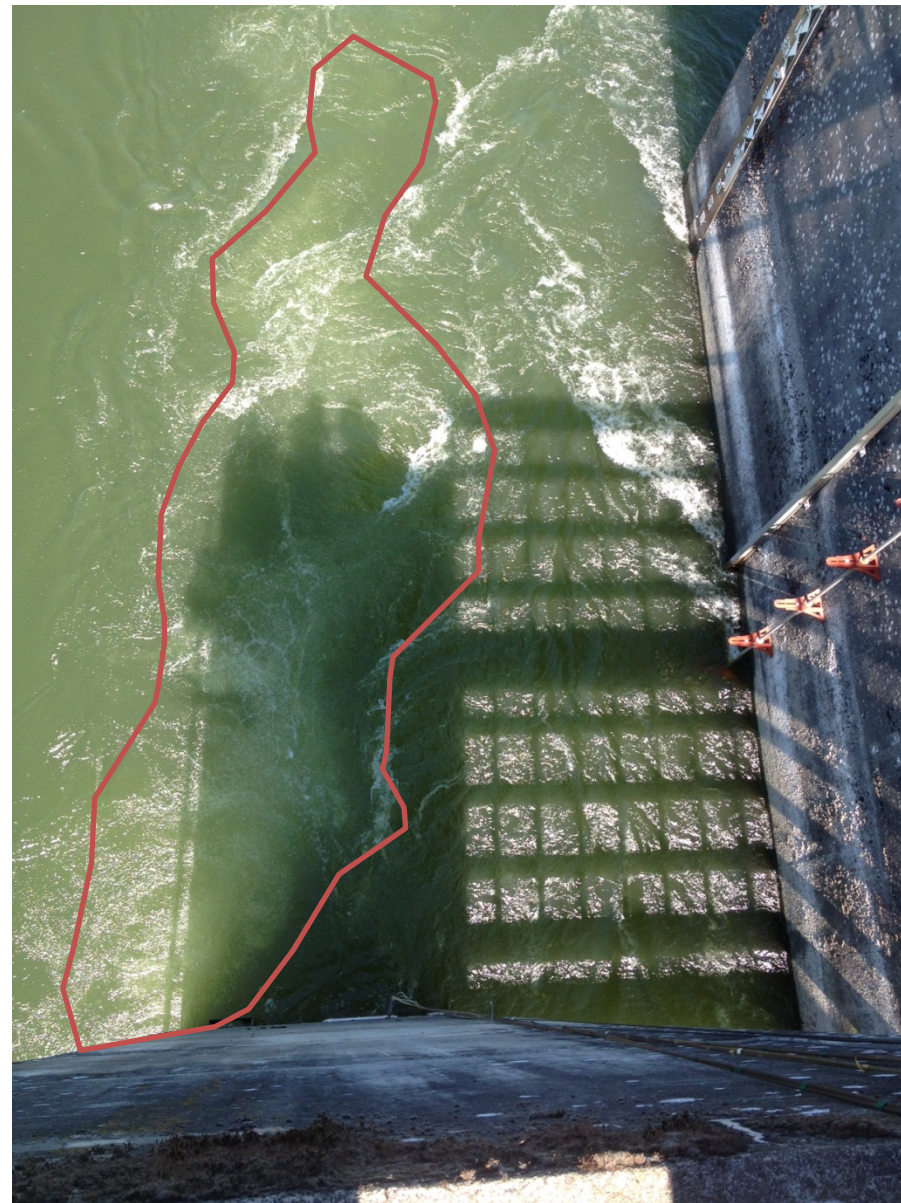
B. 50% valve opening on 7/9/14 (TW = 19 ft). Consistent discharge of entrained air from main flume structure, and intermittent bubble plume from LFS entrances, in vicinity of NDE. Similar to observed pattern on 6/18/14 FPOM site visit.
